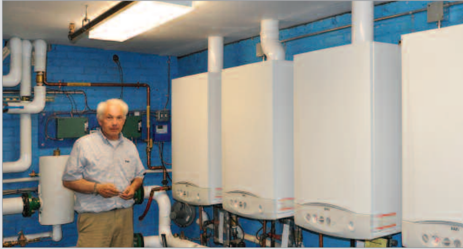
From left to right Installation of high-efficiency Baxi's boilers at Biddeford Ice Arena in Maine (2005).
